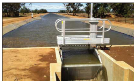
Figure 3 Lined channel section with Rubicon control gates
